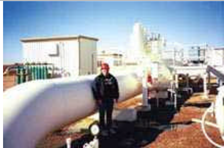
Colorado Experimental Engineering Inc. (CEESI) is equipped to calibrate many types of flowmeters and valves.
