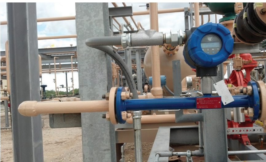
Here a Magnetrol flow-body (spool-piece) type inline sensor measures natural gas for an exploration and production company.
