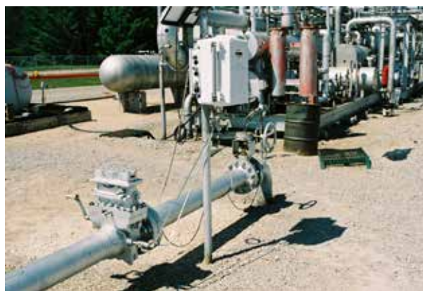
Figure 3. A DP flowmeter installed in an oilfield near Traverse City, Michigan.
