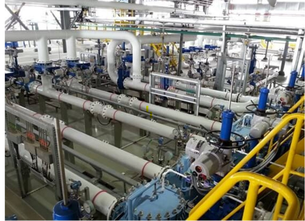
A petroleum liquid processing facility
